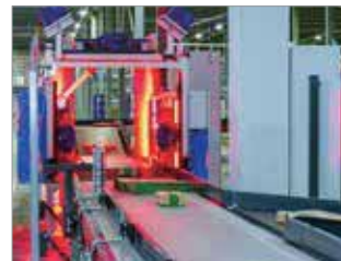
DWS front-end belt conveyor
