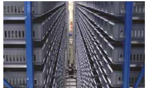
Rail dependent storage and retrieval equipment
